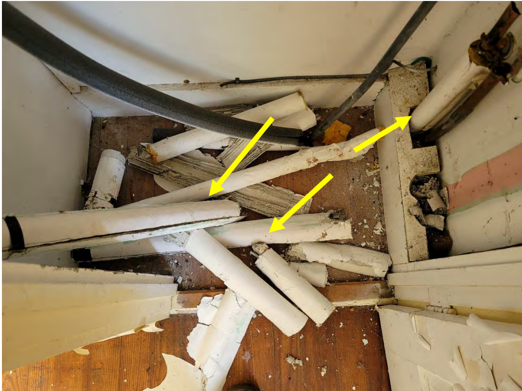
Air cell (ACM) pipe insulation 1 st floor, bedroom 1, closet.
