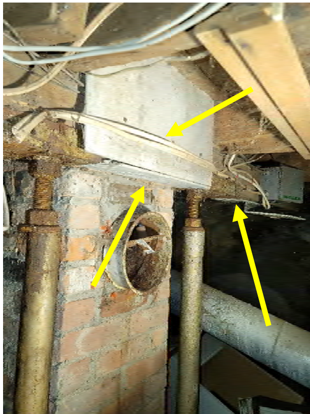
Transite (ACM) board, basement furnace area.
