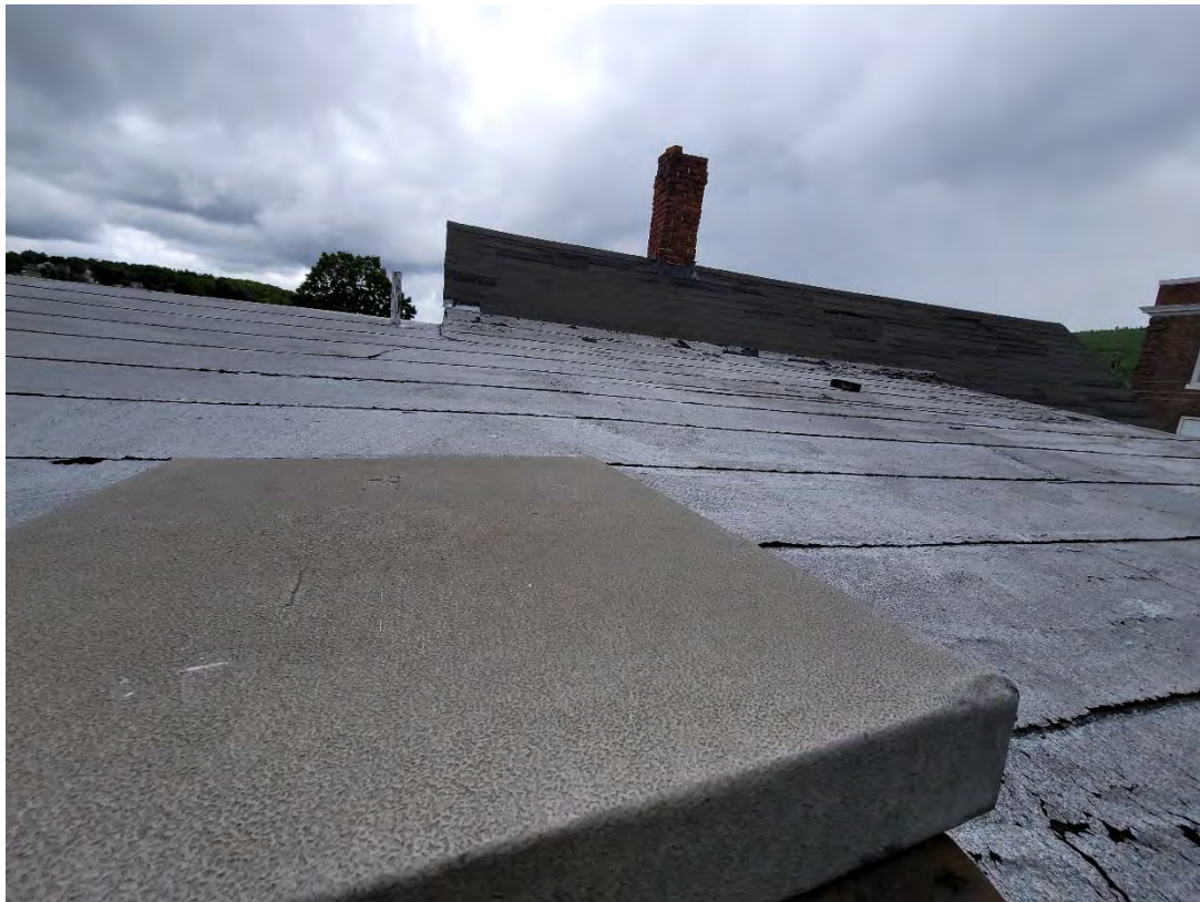
ACM roofing on south porch and "bump out" roof. Roof hatch in foreground.
