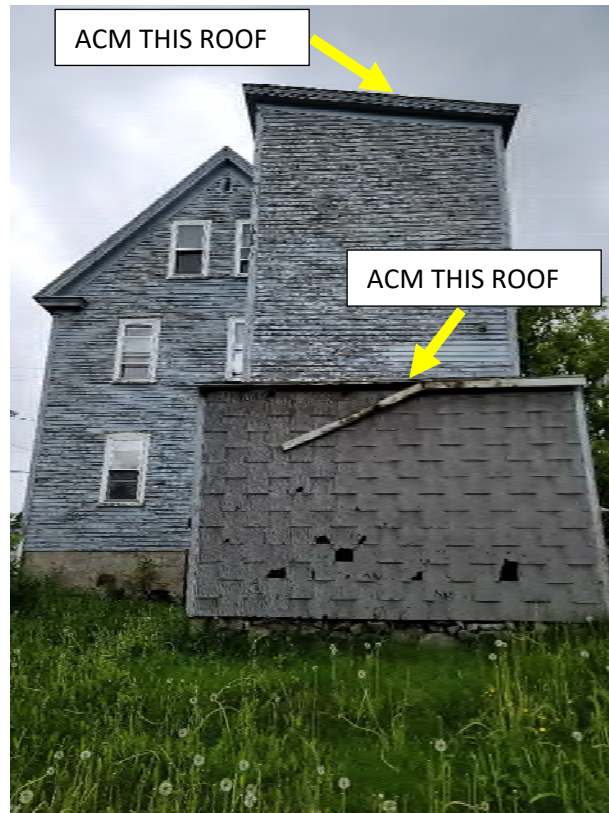
ACM roofing on south porch and "bump out" roof (top) and rear shed (bottom).
