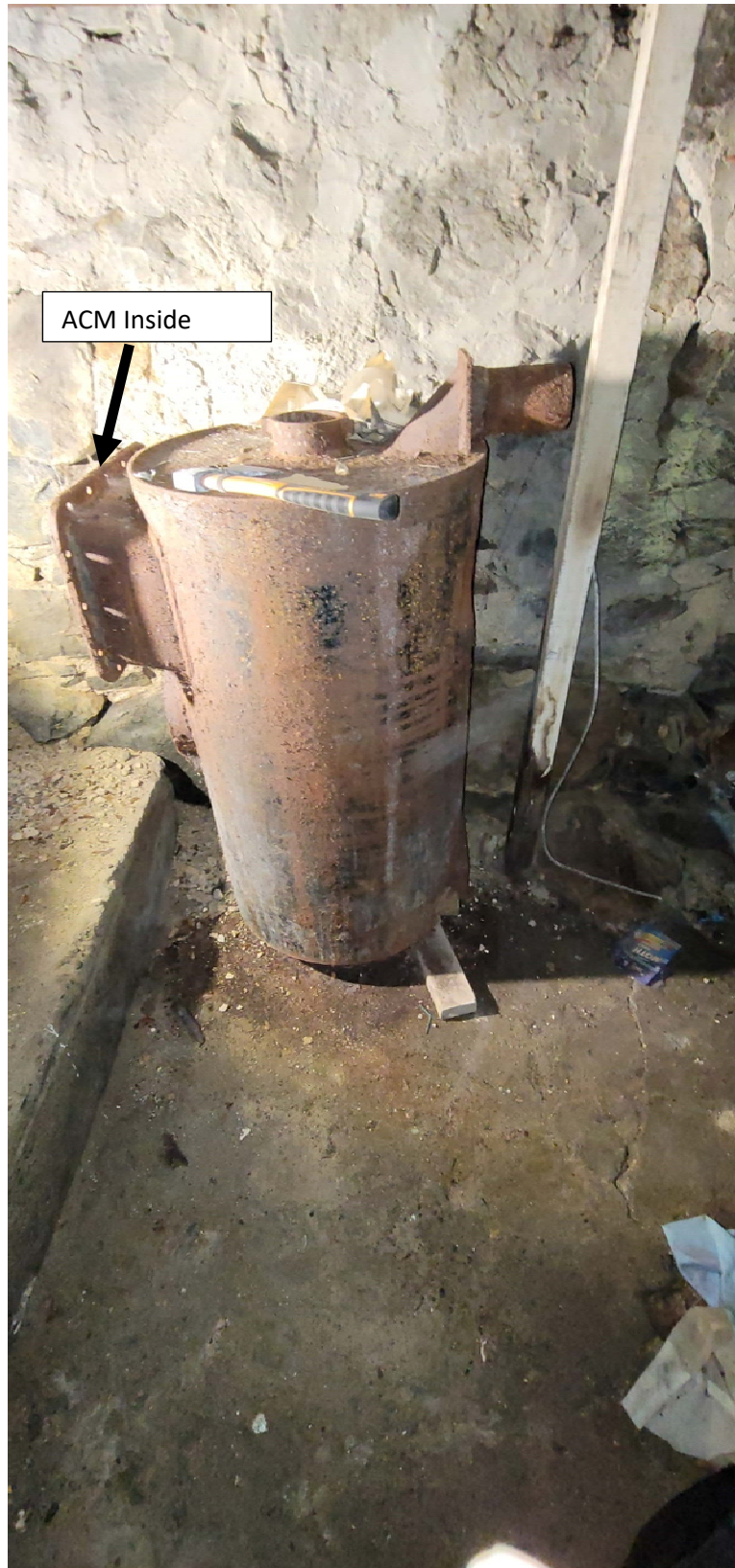
Abandoned Boiler in Basement. Aircell (ACM) Pipe Insulation Remnants Inside (Sample B-3).
