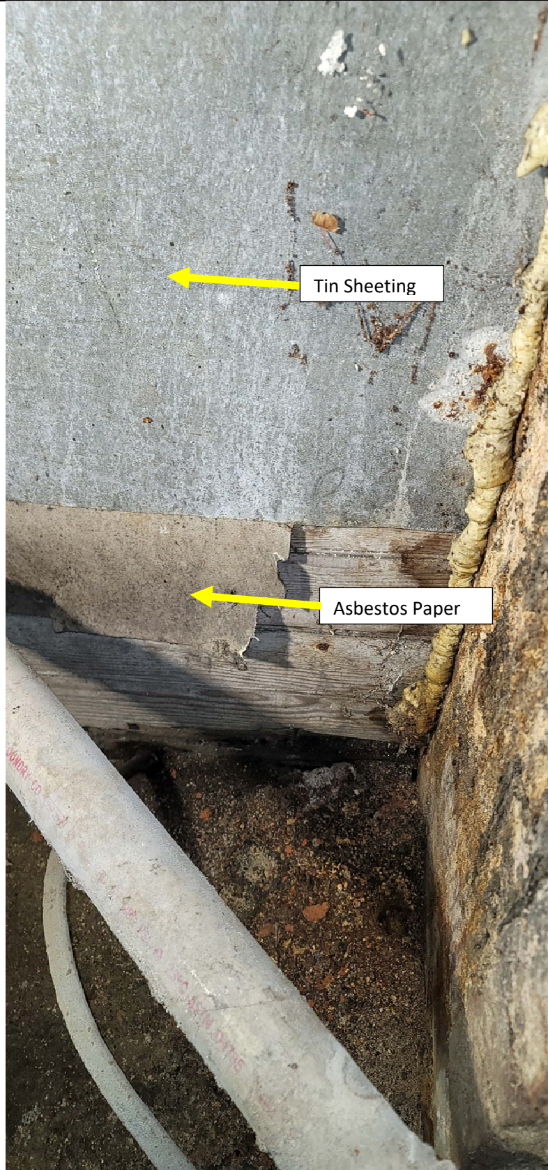
Asbestos Paper (Sample B2) in Basement, Behind Tin Sheetting.
