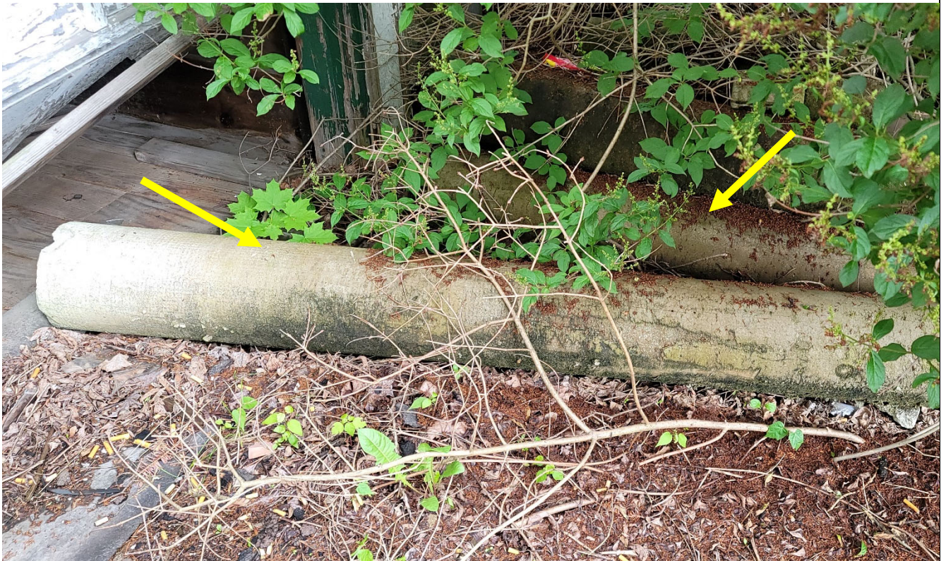
Transite pipe stored outside garage.
